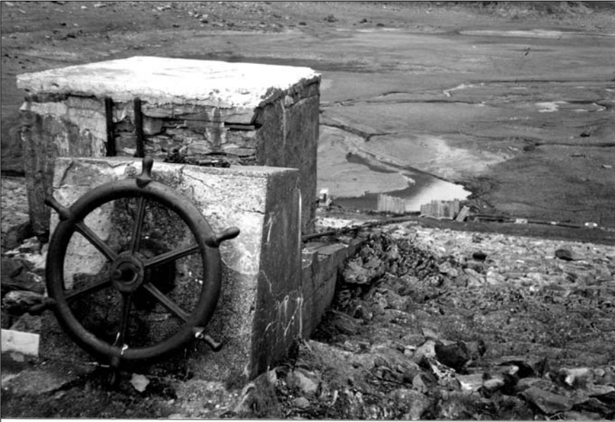
The sluice control in 1996, looking north into the empty reservoir during repairs to the dam by Croppers of Burneside.
